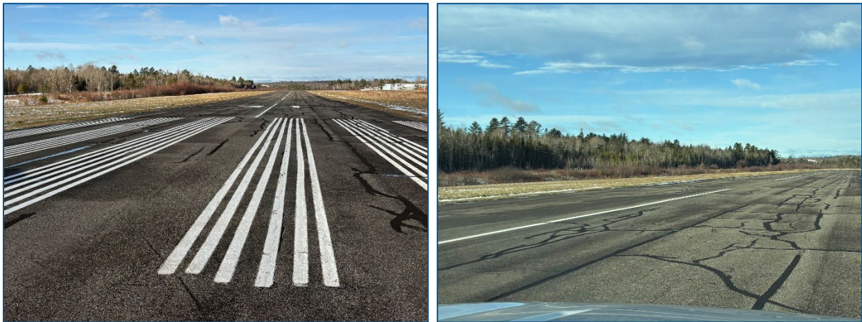
Pavement surface conditions at the Runway 31 threshold (left) and approximate midpoint (right)
