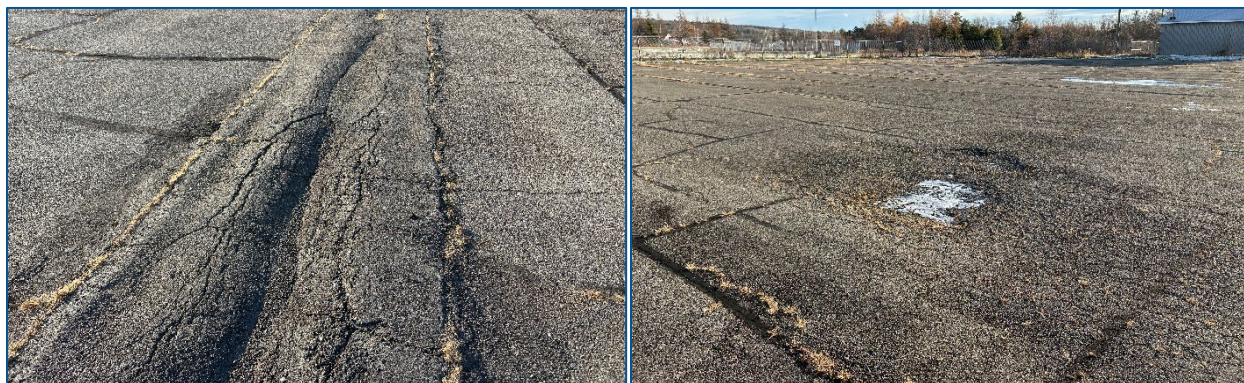
Apron I representative high severity rutting and raveling
